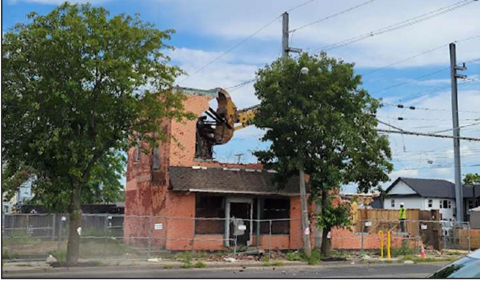
On August 10th city officials commenced with the demolition of the building on Broadway and John St. commonly known by locals as the "Pigeon Palace." The building formerly was the corporate office of the Raritan River Railroad, a police sub-station for both Conrail and NJ Transit Police, and office for a taxi company. The city plans to expand the current parking lot on Broadway between John St. and Henry St. (Photo/Info by Jamie Norek)
